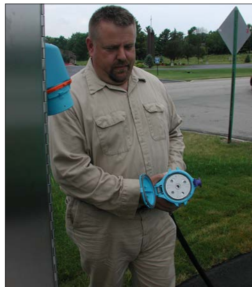
Connecting a generator to the lift station is fast, safe, and easy, and an electrician is not required at the jobsite. When disconnected, the plug's dead-front construction keeps workers safe by preventing accidental contact with live parts.
