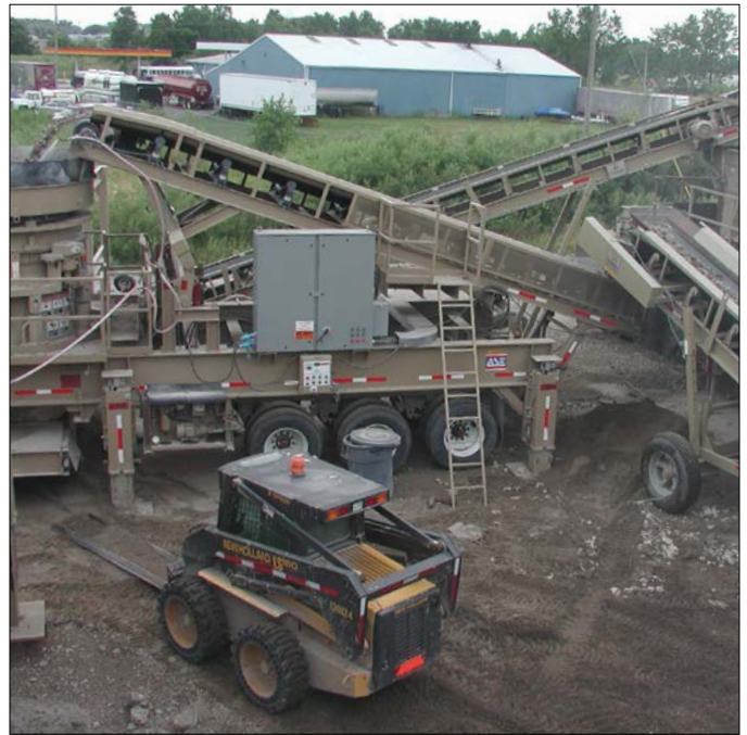
The portable crushing plant is moved frequently, so speed and ease of making power connections is important.
