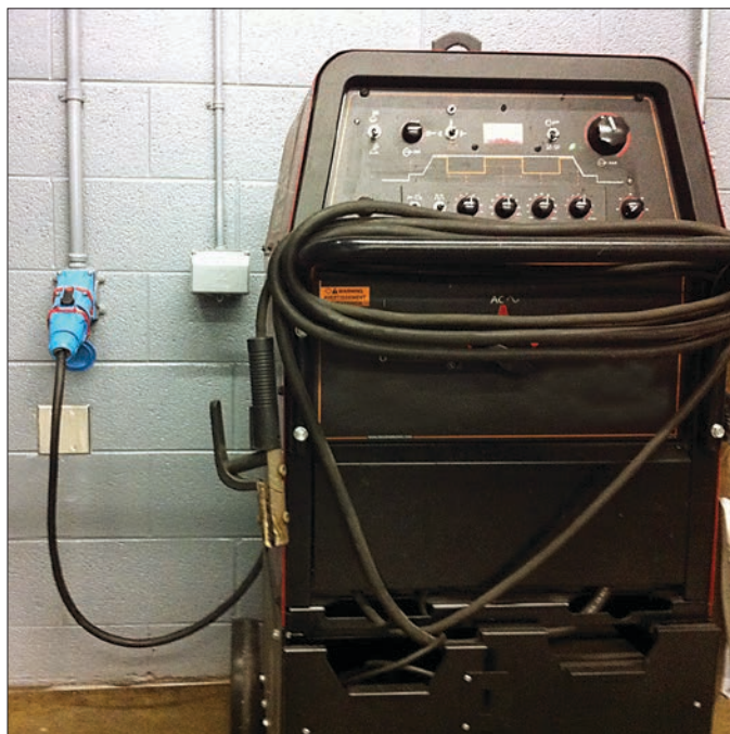
Exclusive safety features make MELTRIC Switch-Rated plugs and receptacles ideal for connecting power to welding machines at Odessa College.
