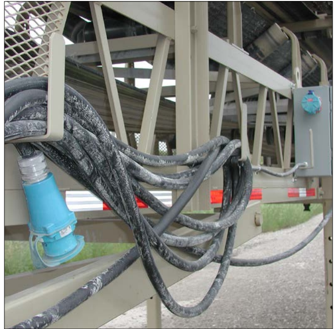
A typical portable conveyor setup includes a MELTRIC plug and connector on panel and power cord. MELTRIC's easy twist connection is not affected by grit like the threaded nut on previous pin-and-sleeve connectors.
