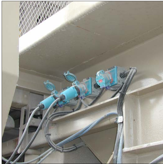
This close up shows multiple MELTRIC connections that facilitate ease of moving portable plant components.
