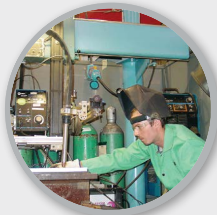
Switch-Rated plug and receptacle (background) enables technician to safely deenergize and relocate welding equipment.
