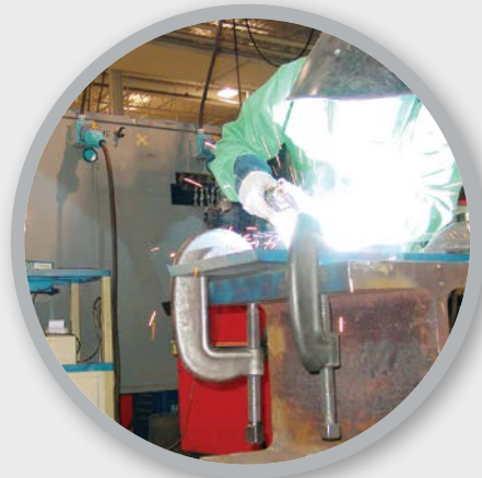
Switch-Rated welding receptacles (background) are connected to overhead busway system via cord drops.
