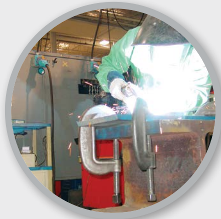
Switch-Rated welding receptacles (background) are connected to overhead busway system via cord drops.
