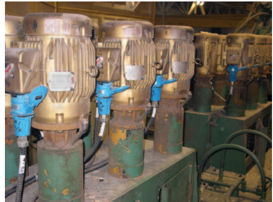
Optimil sawbox at Canfor's Houston, BC mill has 12 motors that must be removed frequently to facilitate routine maintenance. Meltric's switch rated Decontactors (in blue) make the job faster and easier than rewiring each time.
