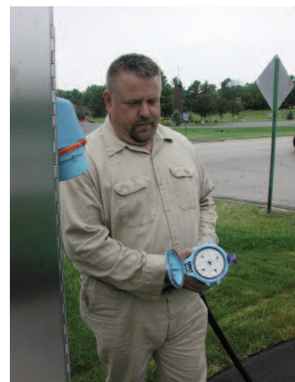
Connecting a generator to the lift station is fast, safe and easy, and an electrician is not required at the jobsite. When disconnected, the plug’s dead-front construction keeps workers safe by preventing accidental contact with live parts.
