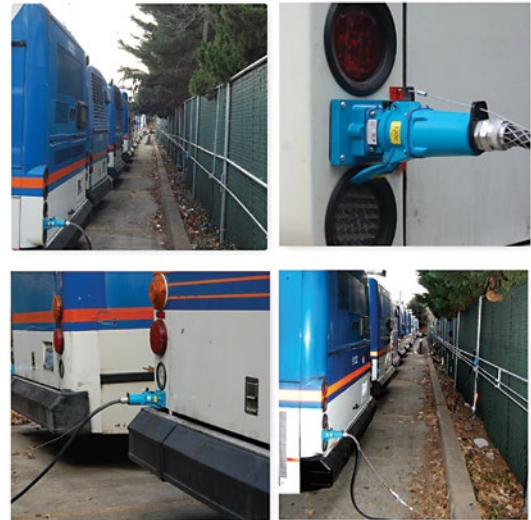
After installing MELTRIC self-ejecting plugs and connectors on its bus fleet, UVA at Charlottesville experienced a steep decline in power plug runaway accidents.
