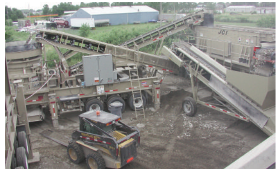
Portable crushing plant is moved frequently, so ease of making power connections is important.
