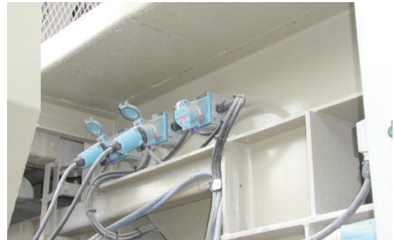
Closeup shows multiple connections that facilitate ease of moving portable plant components.
