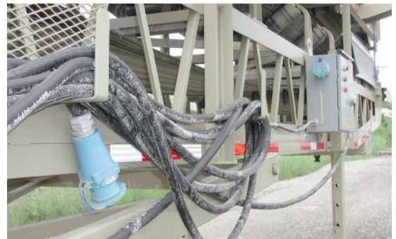
Typical portable conveyor setup includes Meltric plug and connector on panel and power cord. Easy twist connection is not affected by grit like the threaded nut on previous pin-and-sleeve connectors.
