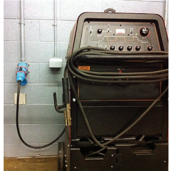
Exclusive safety features make Meltric's Switch-Rated plugs and receptacles ideal for connecting power to welding machines at Odessa College.
