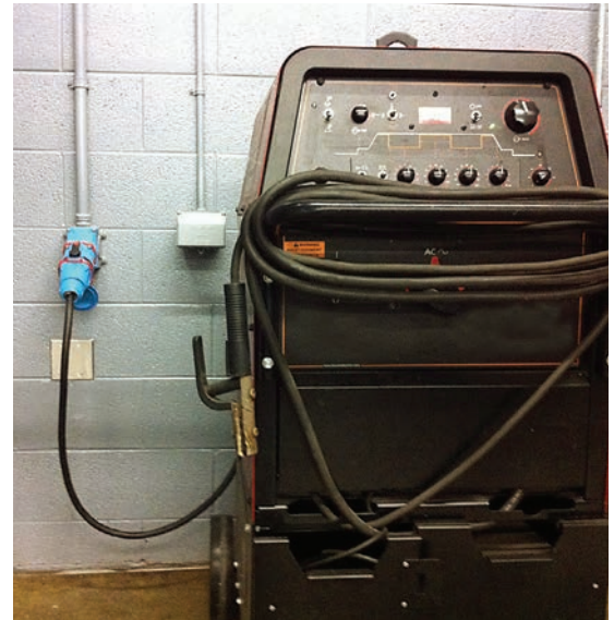
Exclusive safety features make Meltric's Switch-Rated plugs and receptacles ideal for connecting power to welding machines at Odessa College.
