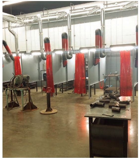
Welding equipment change-outs at Odessa College are simple and safe because the newly installed plugs and receptacles from Meltric protect operators from live parts and arc flash.
