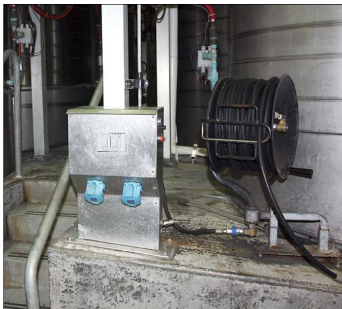
MELTRIC switch-rated plugs and receptacles provide a safe, quick and reliable way to connect and disconnect pumps, bottling machinery and harvest equipment to the 220V 3 phase outlets at ZD Wines.
