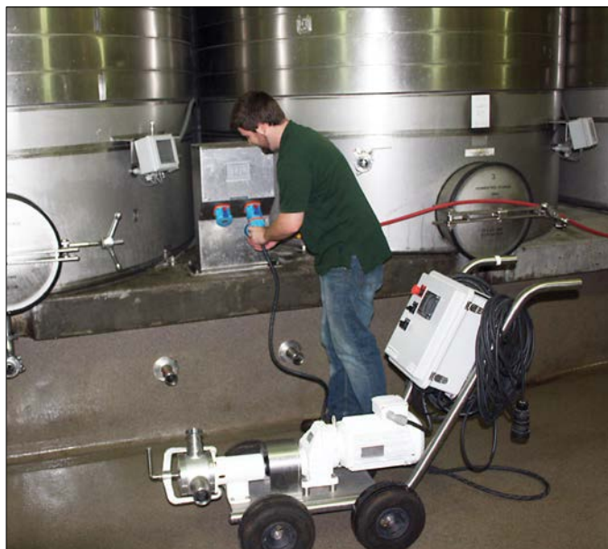
Washing down equipment is a frequent activity at ZD Wines. MELTRIC Switch-rated plugs and receptacles are automatically Type 4X watertight whenever they are mated together.
