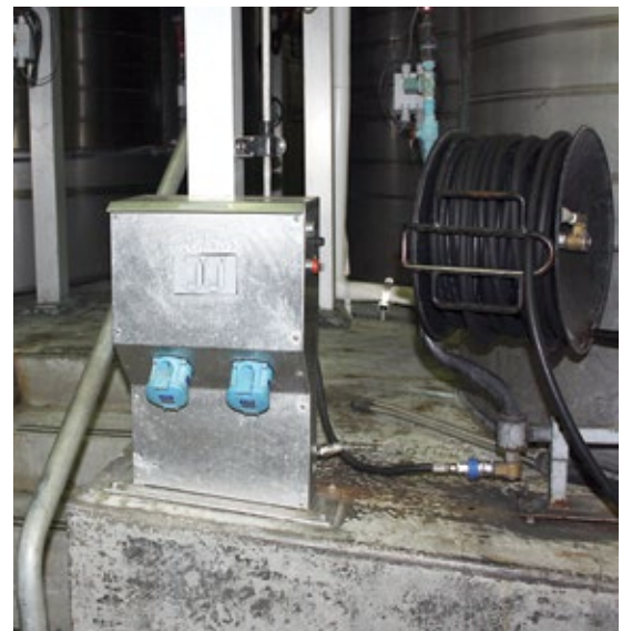
Meltric DECONTACTOR™ Series switch-rated Plugs and Receptacles provide a safe, quick and reliable way to connect and disconnect pumps, bottling machinery and harvest equipment to the 220V 3 phase outlets at ZD Wines.
