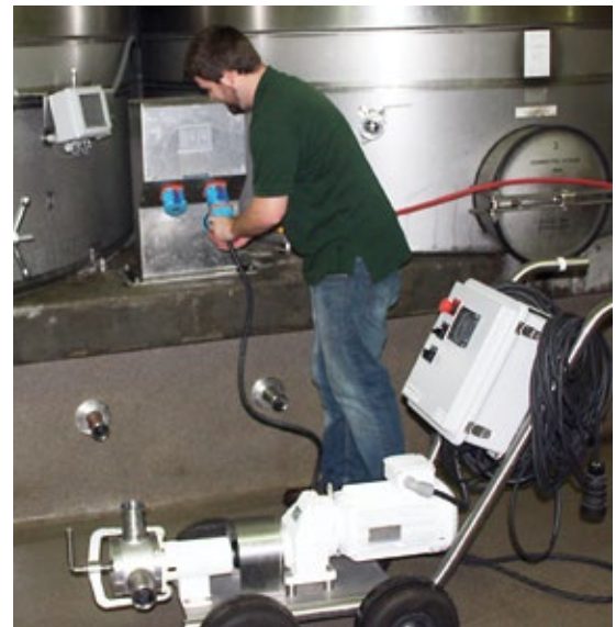
Ryan Carson, Cellar Man at ZD Wines uses Meltric DECONTACTOR plugs and receptacles for their immeasurable amount of safety and plug-n-play capability, which reduces time spent connecting and disconnecting portable pump carts.
