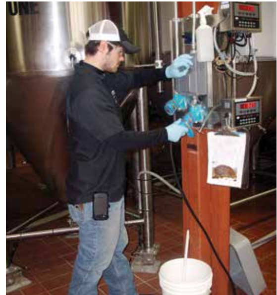
Meltric Decontactor plugs have a modular design and flexible mounting accessories allowing them to be used in a variety of configurations including, in-line, cord drop, or wall mounting. Decontactors are UL and CSA rated for 'motor circuit' and 'branch circuit' disconnect switching and are an approved NEC/CSA 'line of sight' disconnect switch.
