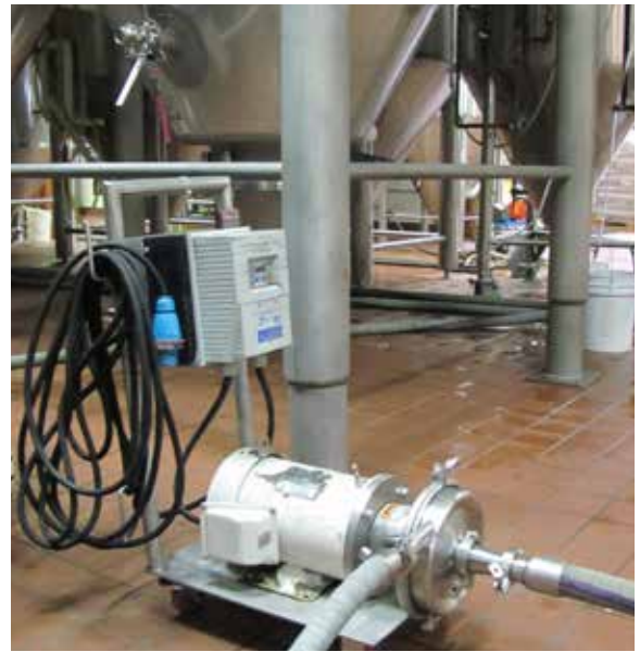
Founders Brewery uses Meltric Decontactor Series switch-rated plugs and receptacles on brewery production equipment such as mobile pump carts, keg washers, motors and other portable equipment. Any qualified worker can connect or disconnect a plug. Making and breaking connections with Decontactor plugs is a Risk Category '0' operation so the need for the cumbersome PPE when working near live parts is eliminated.
