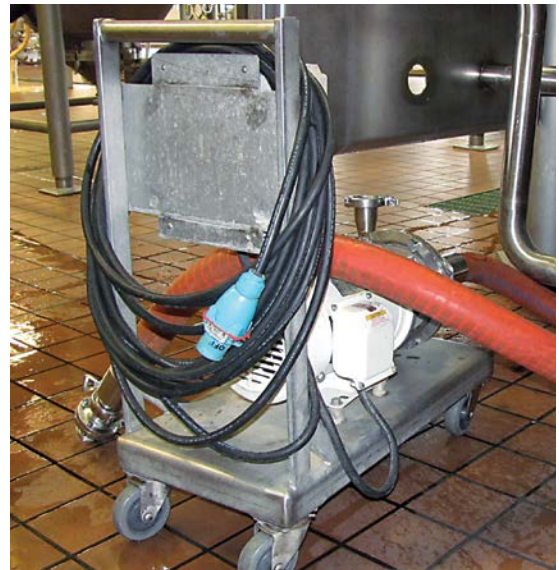
At Bell's Brewery, portable pump carts are connected with Meltric DecontactoRs which combine the safety and functionality of a disconnect switch with the convenience of a plug and receptacle. Their integral switching mechanism allows users to safely make and break connections under full load and provide significant protection in overload and short circuit conditions.
