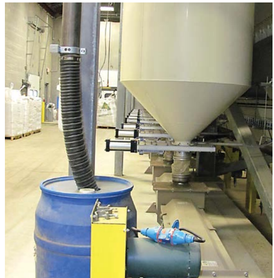
Bell's Brewery has the benefit of limiting downtime on their grain handling equipment, associated with maintenance and motor change-outs, since no hardwiring of connections is necessary.
