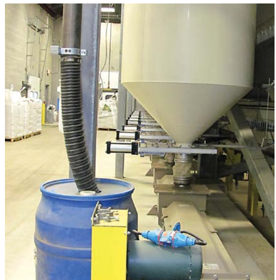
Bell's Brewery has the benefit of limiting downtime on their grain handling equipment, associated with maintenance and motor change-outs, since no hardwiring of connections is necessary.
