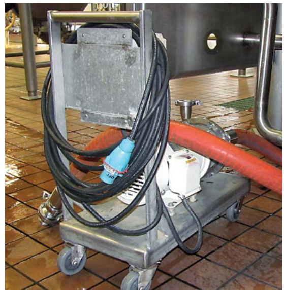
At Bell's Brewery, portable pump carts are connected with Meltric Decontactors which combine the safety and functionality of a disconnect switch with the convenience of a plug and receptacle. Their integral switching mechanism allows users to safely make and break connections under full load and provide significant protection in overload and short circuit conditions.
