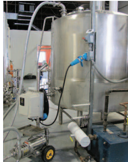
Portable pump carts are connected with Meltric Deconnectors for their immeasurable amount of safety and plug-n-play capability, which reduces time spent connecting and disconnecting frequently moved equipment.
