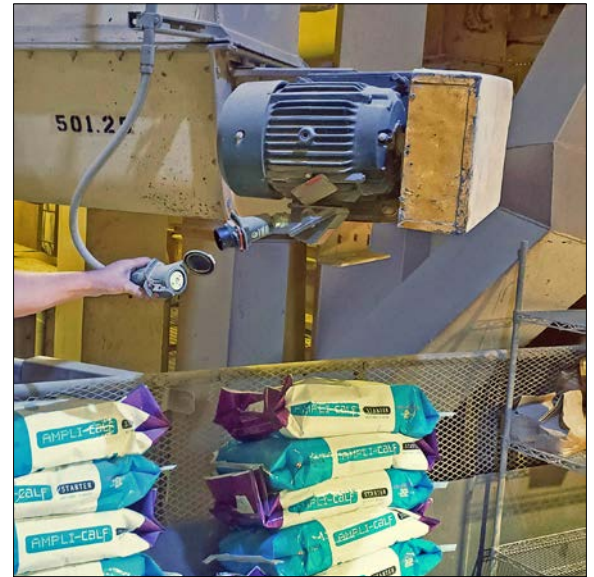
Purina Mill uses MELTRIC DXN Hazardous Location plugs and receptacles for motor connections throughout their plant. Plug and play connections simplify motor maintenance and changeouts.
