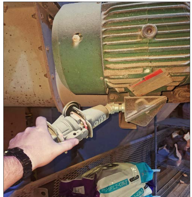
Safe, push-button deenergization simplifies motor and equipment changeouts. This improves efficiency and minimizes downtime.
