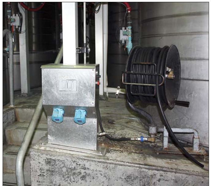
MELTRIC Switch-Rated plugs and receptacles provide a safe, quick and reliable way to connect and disconnect pumps, bottling machinery and harvest equipment to the 220V 3 phase outlets at ZD Wines.
