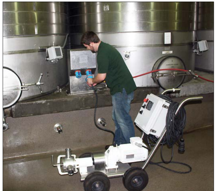
Washing down equipment is a frequent activity at ZD Wines. MELTRIC Switch-Rated plugs and receptacles are automatically Type 4X watertight whenever they are mated together.
