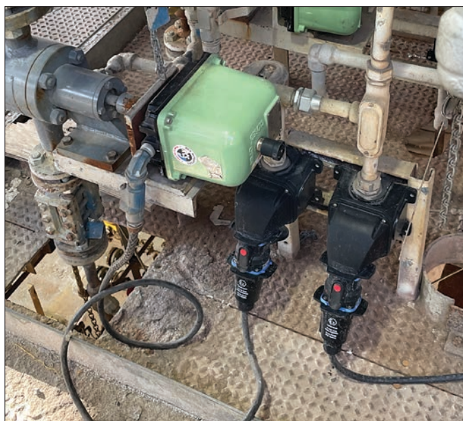
MELTRIC DXN Hazardous Location plugs and receptacles being used on critical equipment.
