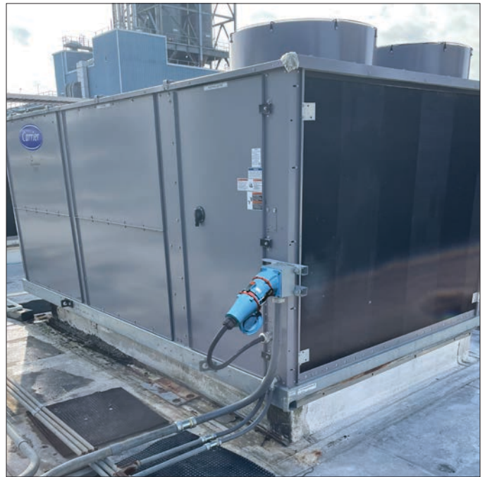
HVAC equipment installed with a MELTRIC Switch-Rated plug and receptacle.
