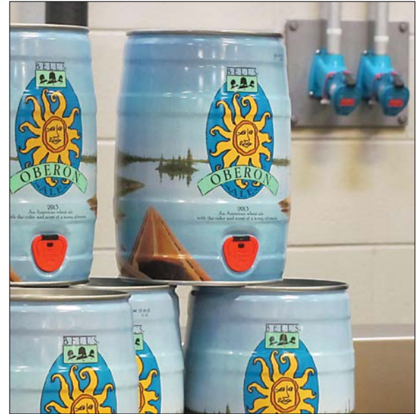
MELTRIC Switch-Rated plugs and receptacles are favored by Bell's Brewery for their safety, reliability, and ability to reduce downtime during maintenance and motor changeouts.
