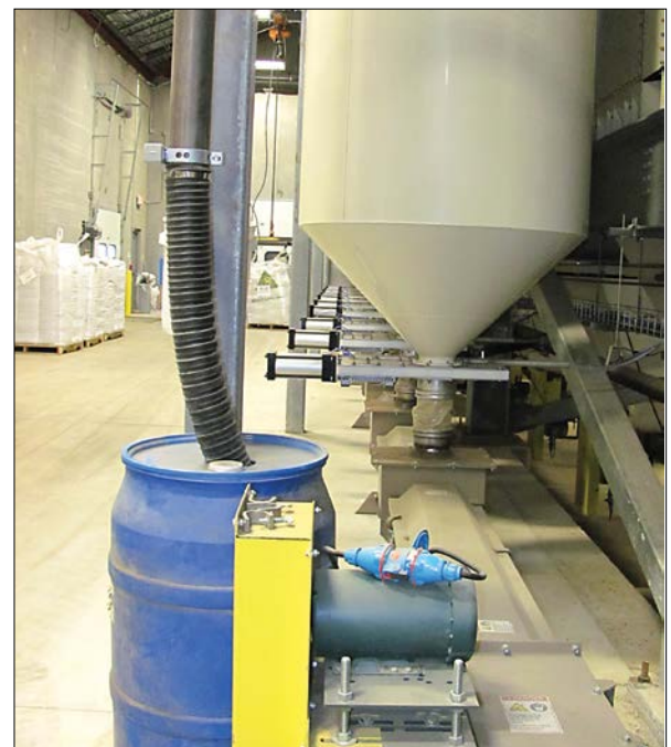
With MELTRIC, hardwired connections aren't necessary. This reduces maintenance and motor changeout downtime for Bell's Brewery.
